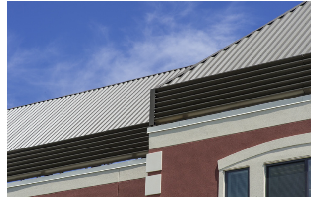
Louvers and a false mansard roof acts to screen rooftop mechanical equipment
